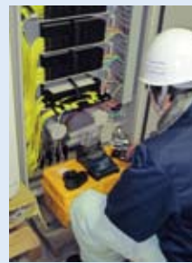
Splicing in ODF
